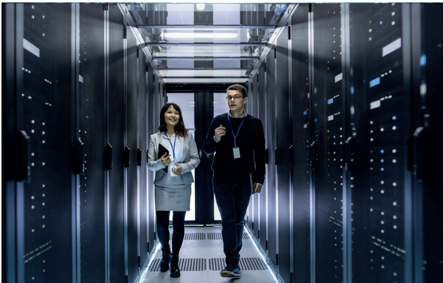
▲ Data centre installation
